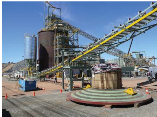
Figure 4: Crusher and fine ore bin assembly. Mill end in foreground.
